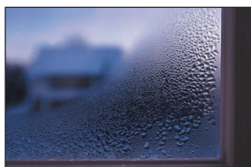
Condensation on the inside of a windowpane.
