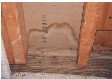
Water stain on a basement wall — locate and fix the source of the water promptly.
